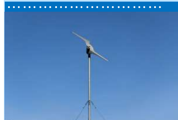
Stand-alone installation on a tower
