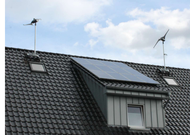
Decoupled roof-top mounted SkyWind NG turbines
