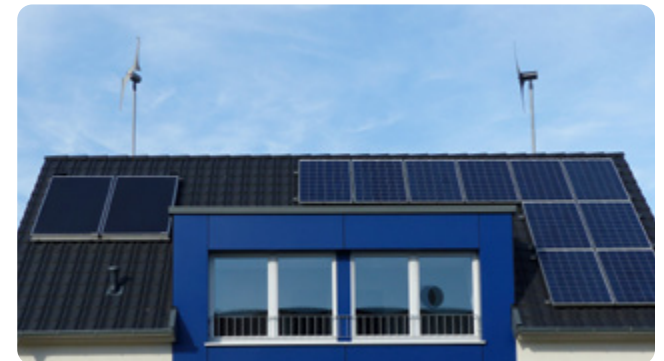
Mounted on a standard rooftop
